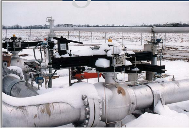
The Gevalco "Emergency Shutdown" module is designed to provide reliable self-contained automatic control of pipeline valves based on emergency conditions.
